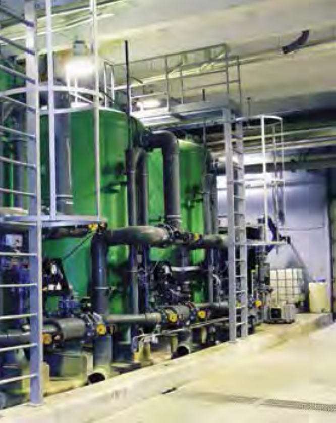
Figure 2.34 Chlorine and waste water tanks in a tertiary water treatment plant.
